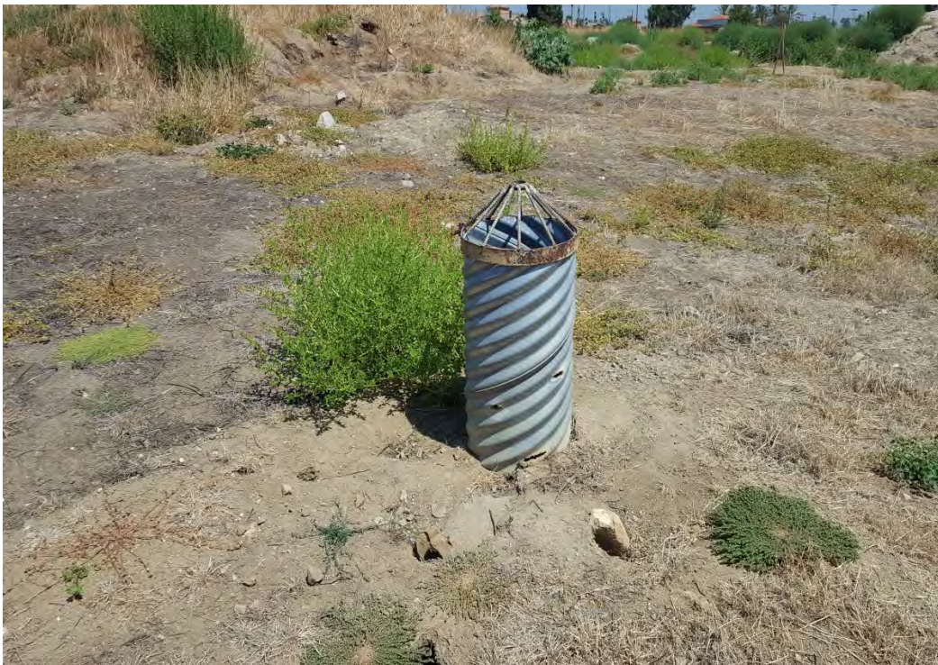
Photo 8. Engineered Drainage Collection Unit in the Central Portion of the Property.
